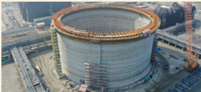
▲ Completion of the slip form with an elevation of 28m at the exterior storage. Currently, pre-cast construction and interior storage welding are in progress.
